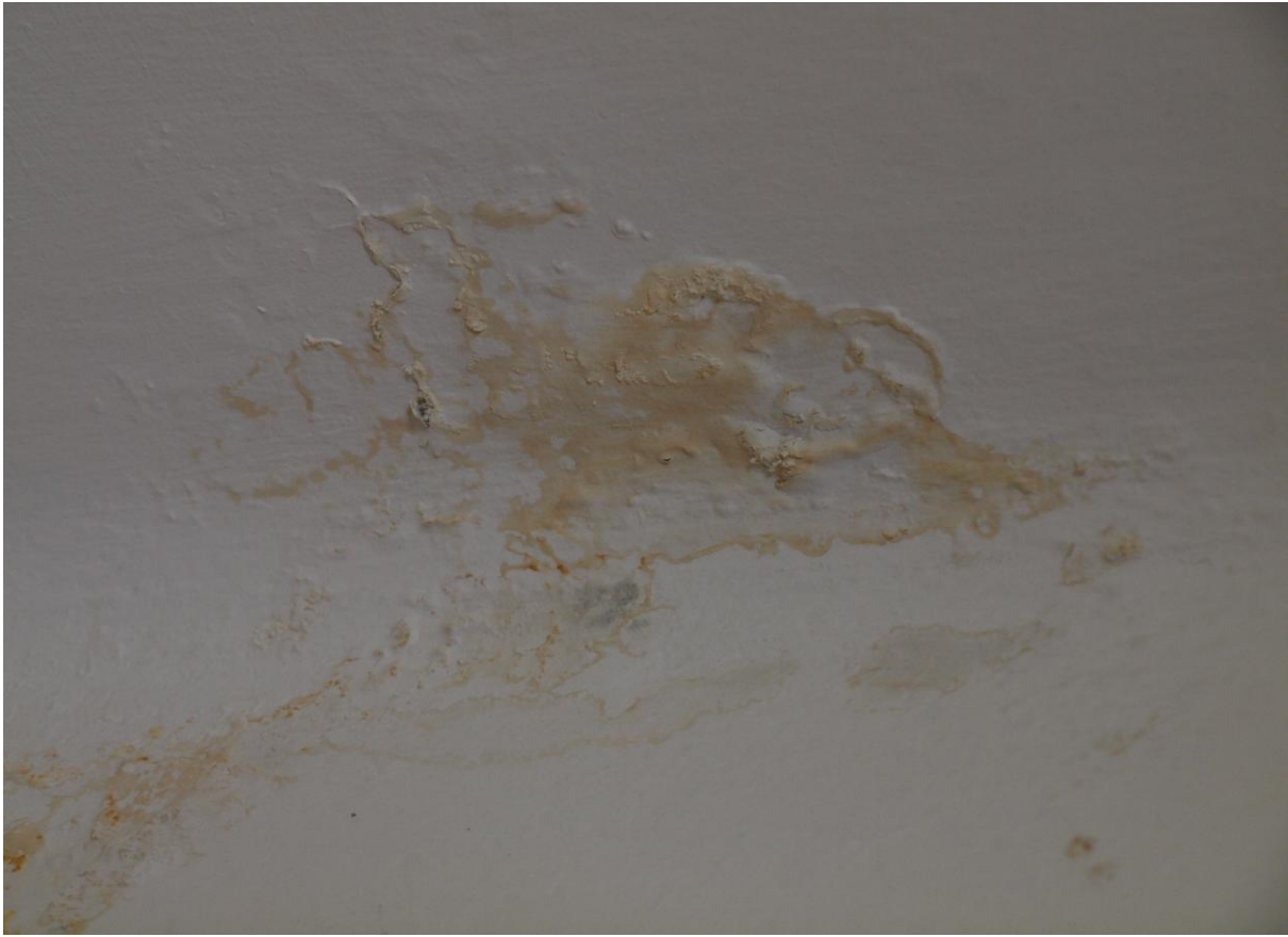
Figure 3. Another example of damage: the plaster layer is peeling off in blisters and flakes, emitting dirt and probably CFUs (again the green shades). The wall and ceiling should be explored till firm layers undamaged by water. Difficult to perform with collections remaining in the room; this problem however was solved couple of years later.
