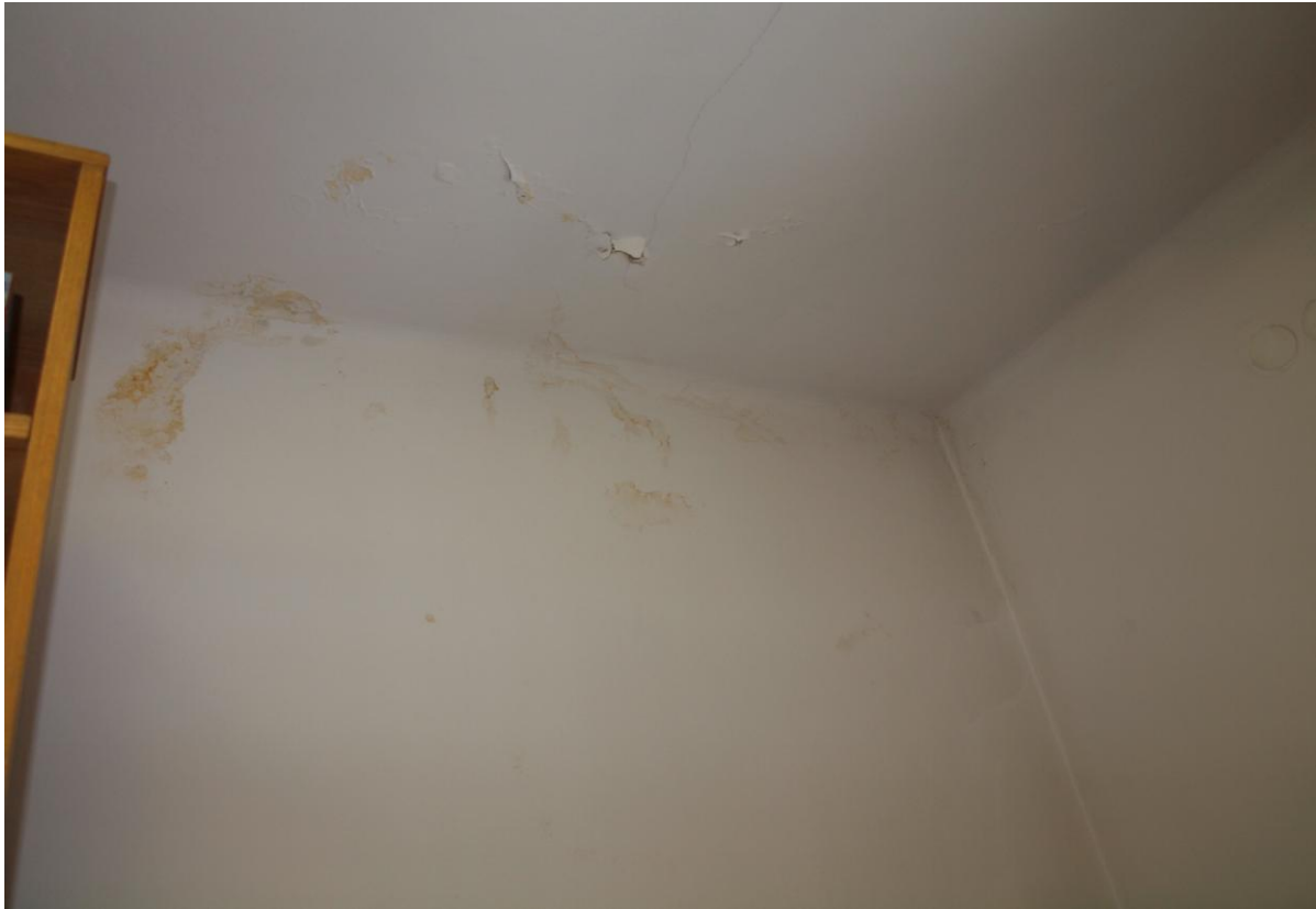
Figure 1. The bookcase in the storage room 218 is already removed and walls and ceiling does not look like heavily damaged. But any repair would require introducing the repair team and a lot of dust while removing the damaged layers of the wall probably down to the bricks.
