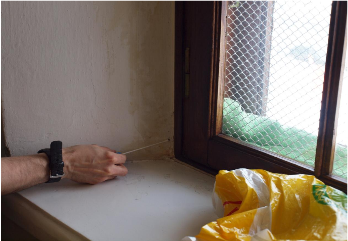
Figure 4. Collecting a dry swab from the window area. Note the evidence of humidity by the window frame and the ad hoc counter action - towel between outer and inner window. Today we have already new windows.
